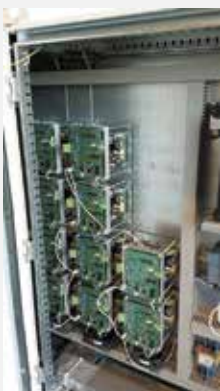
Chopper in armadio, funzioni pulsato e inversione Chopper on rack with pulse plating function and reverse
